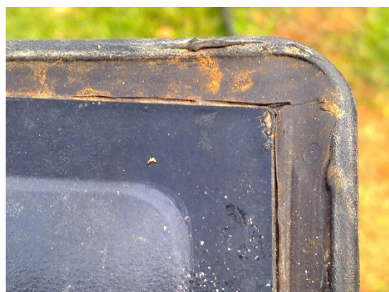
Figure 2: Degradation of the bond between glass cover and collector frame
