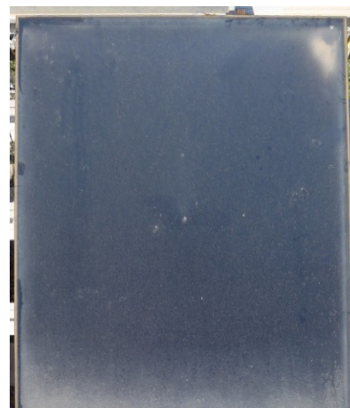
Figure 3: Collector with caked-on dirt on the cover and dirt entry through a pipe penetration
